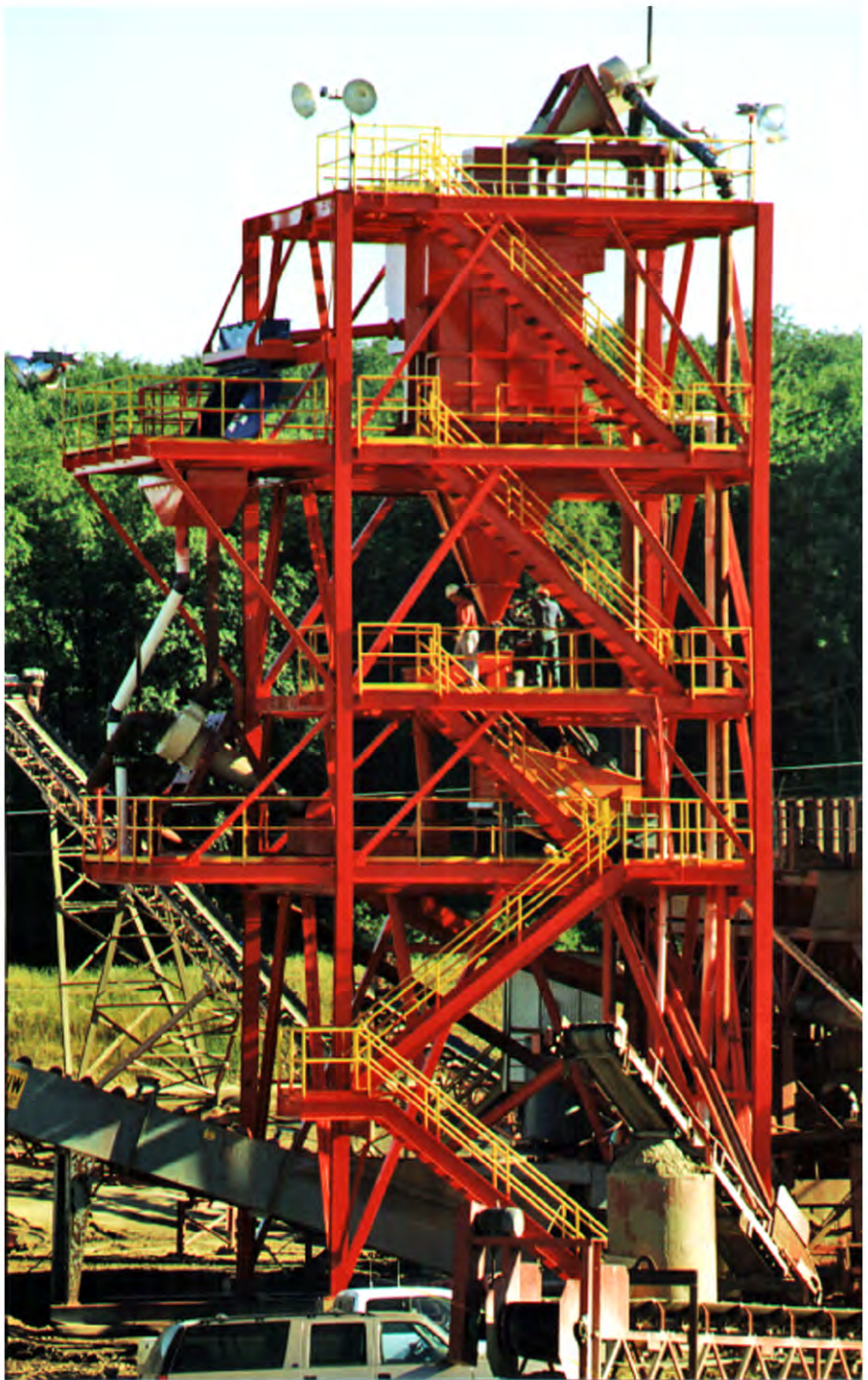
CFS's lignite removal system in operation at G.L. McKnight Sand and Gravel in Slippery Rock, Pa.
